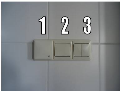
Schakelaars in badkamer
